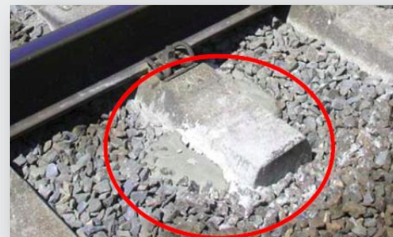
Deterioration of Sleepers and Ballast
