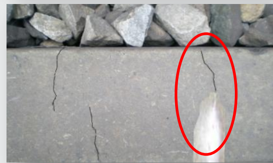
Cracks in Concrete Bearers
