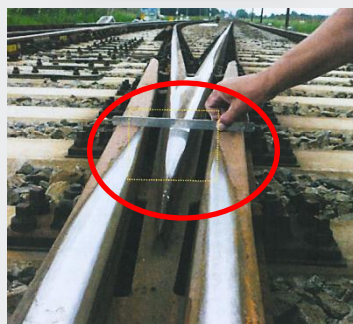
Deterioration/Settling Crossing Nose
